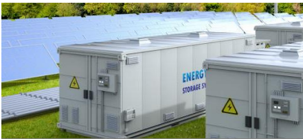
SLOCUM BATTERY ENERGY STORAGE
